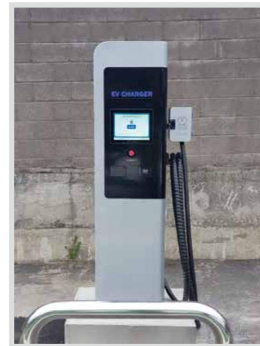
12.1" Panel pc installation in Jeju Island
