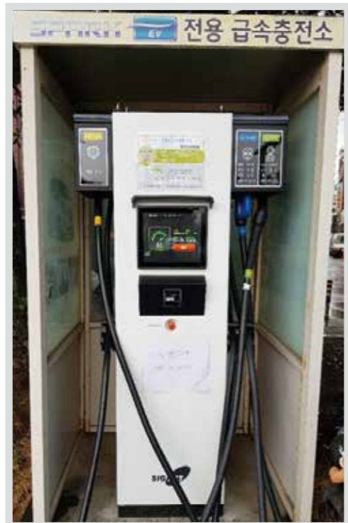
12.1" Panel pc installation in Jeju Island
