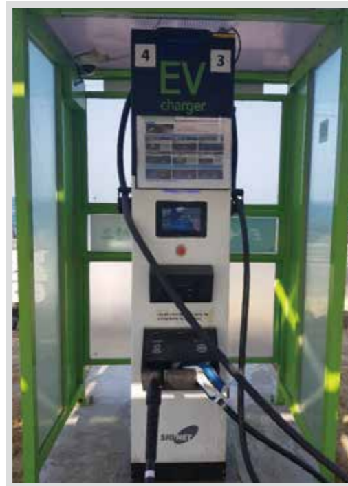
8" Panel pc installation in Jeju Island
