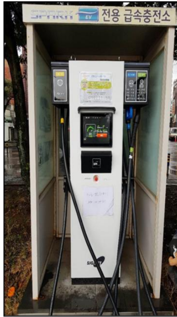
SK Signet Fast charger in Jeju Island ( 15" PANEL PC Applied)
