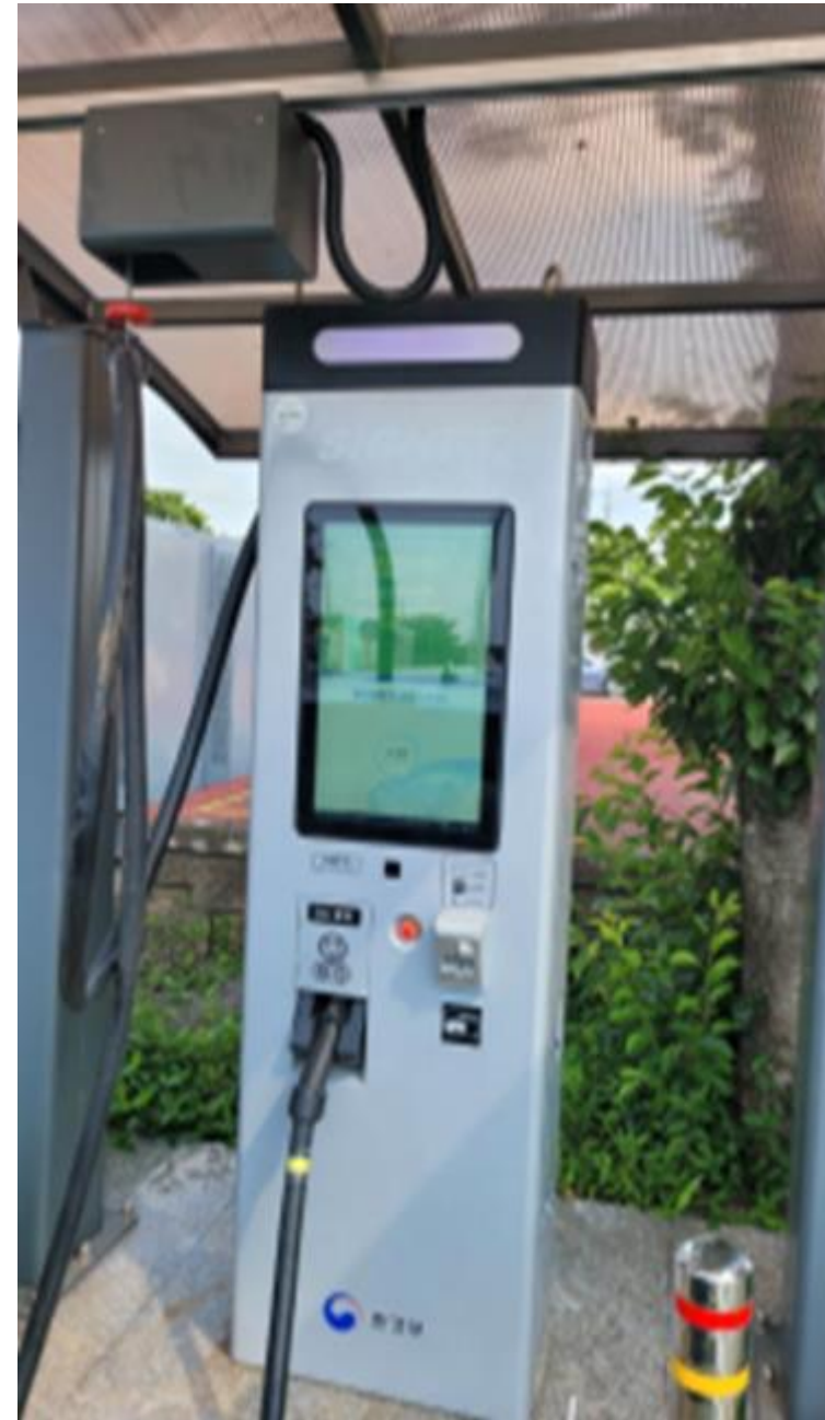
Ministry of Environment Fast charger in Jeju Island ( 24" PANEL PC Applied)
