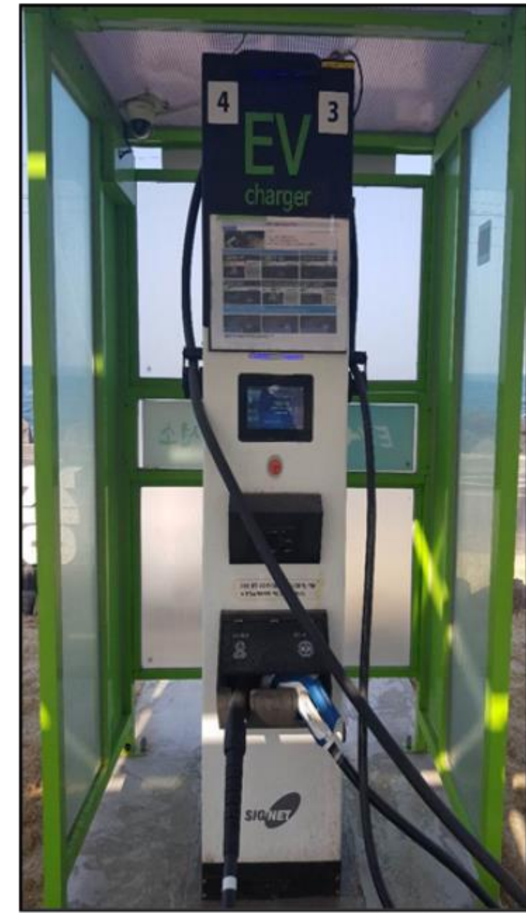
SK Signet Fast charger in Jeju Island ( 12.1" PANEL PC Applied)
