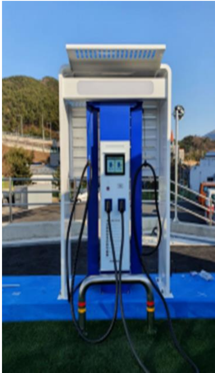
Moderntec Fast charger at busstop ( 12.1" PANEL PC Applied)
